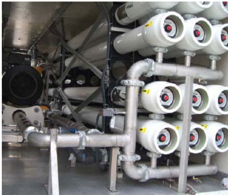
Figure 4 Brine Discharge Piping Using AL-6XN pipe
